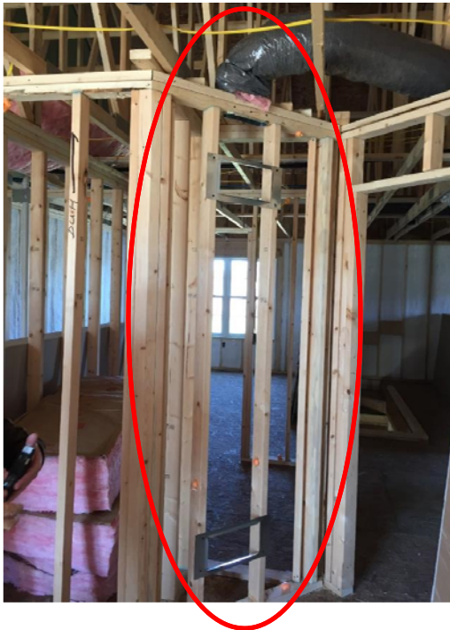
Return air cavity
